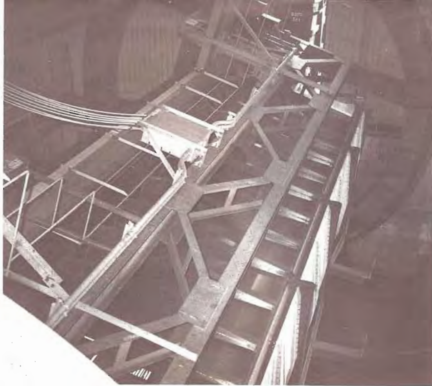
Rotary dumping mechanism at Big Stone Plant overturns each car to empty coal onto open steel grid and through to a conveyor. The grid function is to break apart any large pieces of lignite that may have formed during transit.
