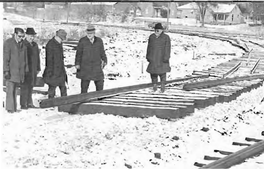
Construction of a turn-out in Bedford, Ind., was started in late February to connect the Milwaukee's main line with that of the Louisville and Nashville Railroad. Inspecting the construction are: (left to right) Division Engineer T. H. Paton; R. L. Tewell, superintendent of the Chicago Terminal—Terre Haute Division; B. J. Worley, vice president-chief engineer; L. V. Anderson, assistant vice president-operation; and Roadmaster Nick Munoz, Terre Haute Division.
