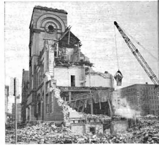
The demolition reveals nostalgic engineering features. Here wrecking crews are ripping into the south elevation.
