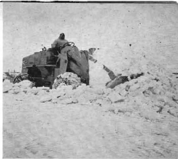
Front end loader operation clears snow-filled cut west of McLaughlin, S. D.
