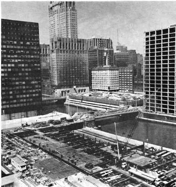
PROGRESS ON GATEWAY CENTER. Scene on the west bank of the Chicago River as work proceeds on Building No. 2 of the office building complex being constructed by Tishman-Gateway Inc. over air rights of the Union Station Company. At right, a
