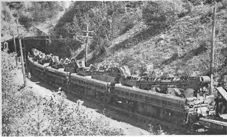
A string of air-dump cars with conveyors for carrying excavated material shown in operation behind a Matisa undercutter machine (out of sight in the tunnel). The cars and conveyor system were specially adapted to this use by the Milwaukee's engineers.
