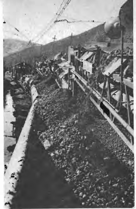
The Matisa train in operation outside the 8,771-foot St. Paul Pass tunnel. Lowering the track in this tunnel at the summit of the Bitterroot Mountains was the largest undertaking in the project.
