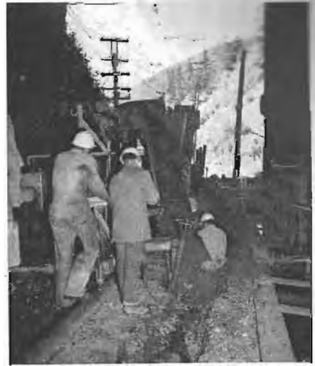
Workmen check the digging chain under the Matisa undercutter. The Swiss-made unit, operating at high speed under the ties, is capable of ripping up 12 inches of material in one pass.
