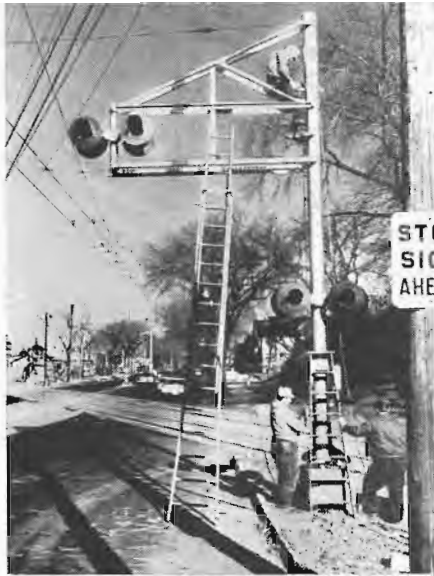
STOP, LOOK AND LISTEN. New automatic grade crossing signals continue to smarten up the scenery along The Milwaukee Road. Pictured completing a recent installation at
