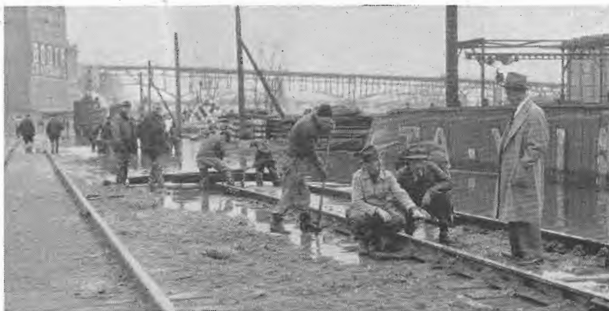
Trainmaster N. H. McKegney indicates depth of water on the Chestnut Street line, St. Paul, when the flood was at its worst. The track at the left has been raised, and the one on which he is standing is in process of being raised. At his left are H. J. Dunn, Twin City Terminal supervisor of telegraph and signals, and F. M. Washburn, district safety engineer (standing).
