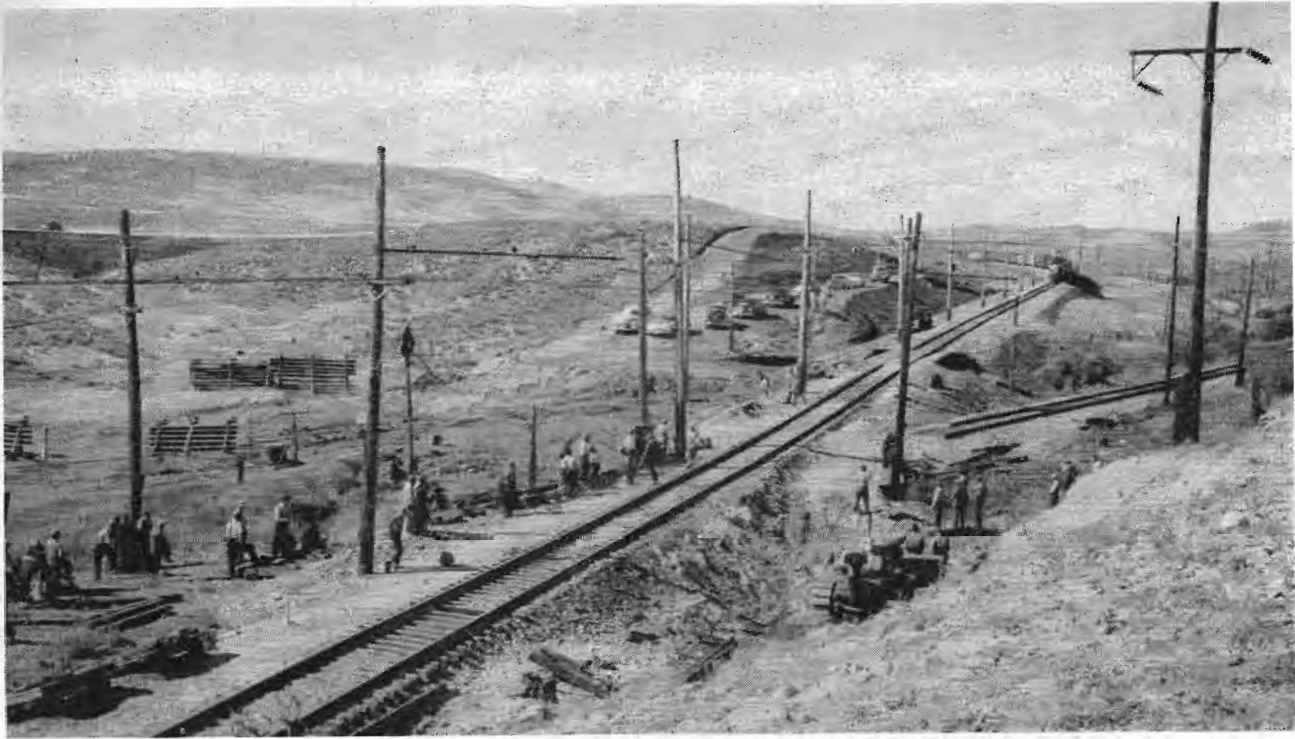
Trackmen step aside as The Milwaukee Road's eastbound transcontinental freight, No. 264, rounds the easy curve at the east end of the new Loweth line on Oct. 3. This was the first train to operate over it. The old line can be seen at right. View is in a westerly direction.
