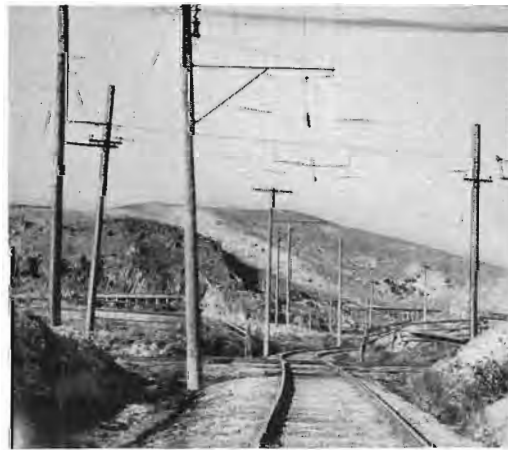
INTERSECTION OF 2400-VOLT SYSTEM WITH TROLLEY CROSSING
